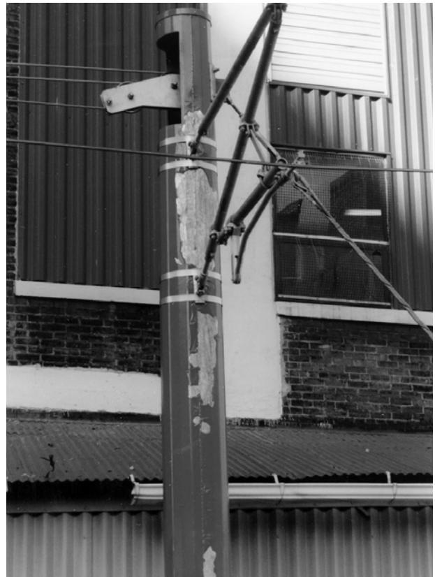
Fig. 5 - Galvanized Pole with Peeling Paint
